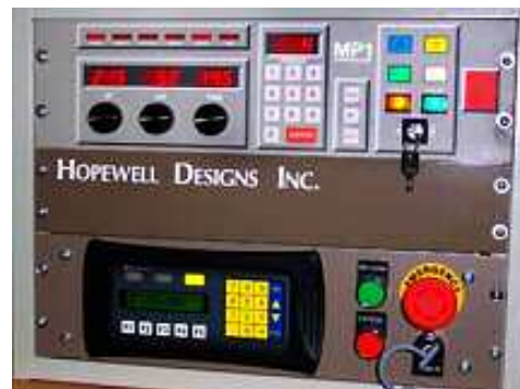
X-Ray and Irradiator Control Panels
