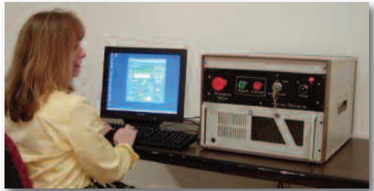
Computer Control Panel
